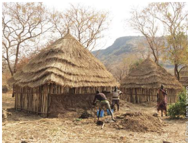
South Sudanese refugees in Tierkidi camp in Gambella, Ethiopia, plastering the walls of the shelters with mud sourced locally by themselves, in areas agreed with authorities and host communities.
