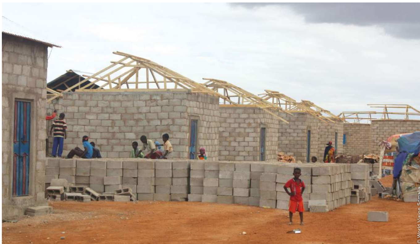
The project built 1,200 permanent houses with accompanying infrastructure across two new sites (here, the site in Garowe).
